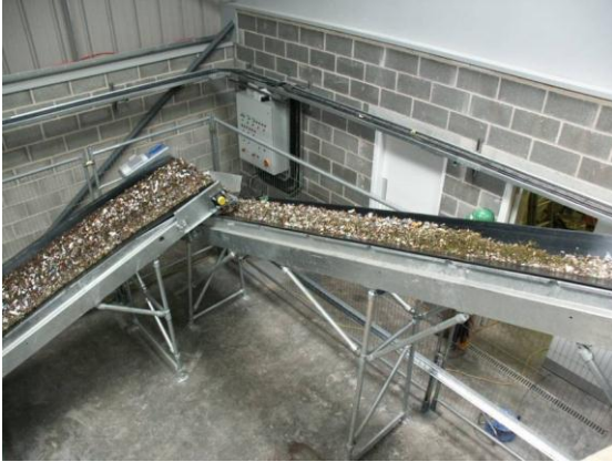
Figure 4.2.2 Reception hall conveyors
